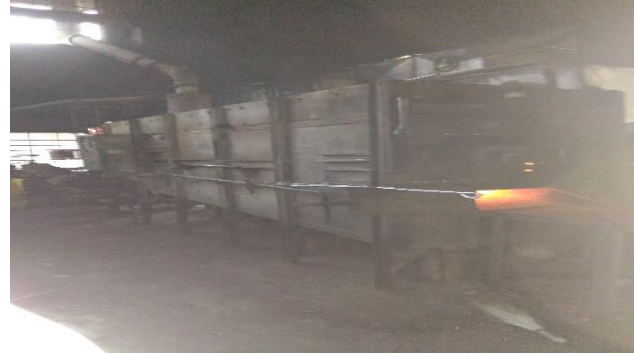
Figure 4: FO Fired Reheating furnace
